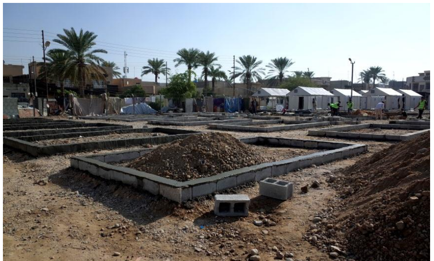
Constructions works in Al Khadra camp in Baghdad. UNHCR recently replaced the 105 tents that had been damaged by the floods in October by refugee housing units. UNHCR/N. Micevic
