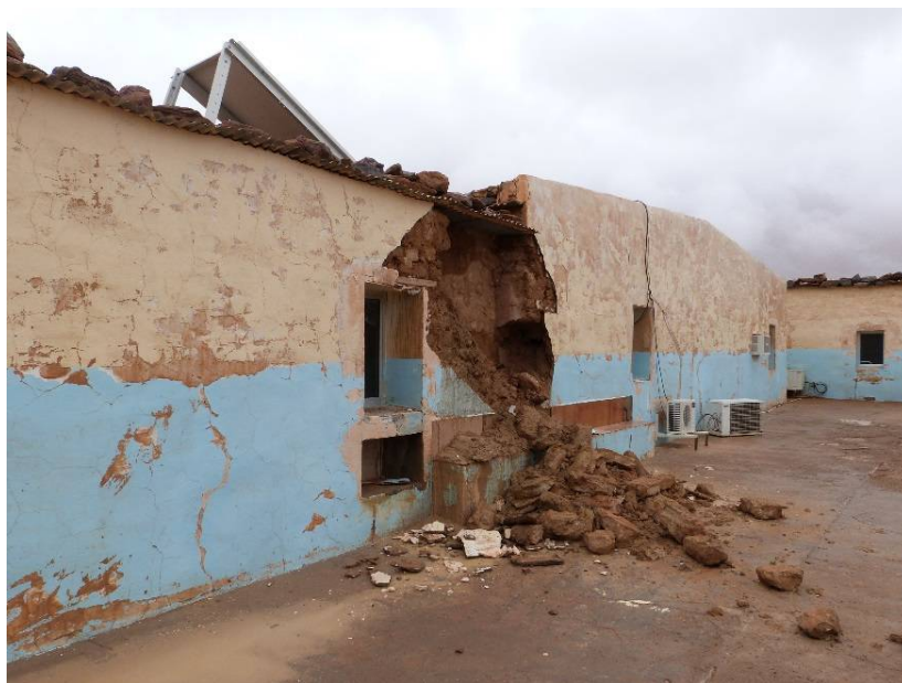
Figure 3: Structural damage to pharmacy, Dakhla camp. Triangle génération humaine/C.Baudoin
