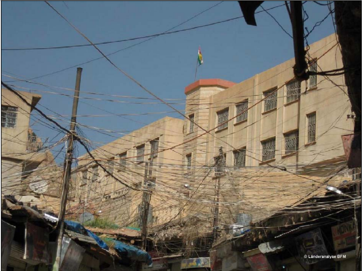
Electricity net in Akre.
