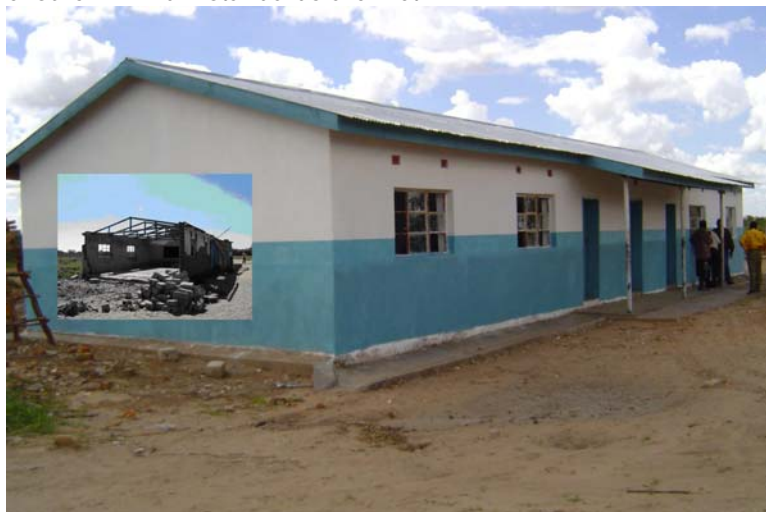
Above, a 1x2-classroom blocks that has undergone rehabilitation at Ngundi Middle basic school. The insert in the above picture depicts the dilapidated building before ZI. Teachers' houses rehabilitation has been completed. The project is funded under Danish embassy small grant contribution to the ZI.
