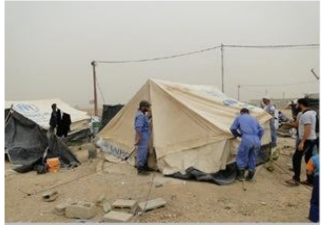
Repairs to storm-damaged tents being carried out at Al Obaidy camp. ISHO/A.Murad
