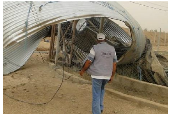
Camp management assess storm damage at Al Obaidy camp. (ISHO/A. Murad)
